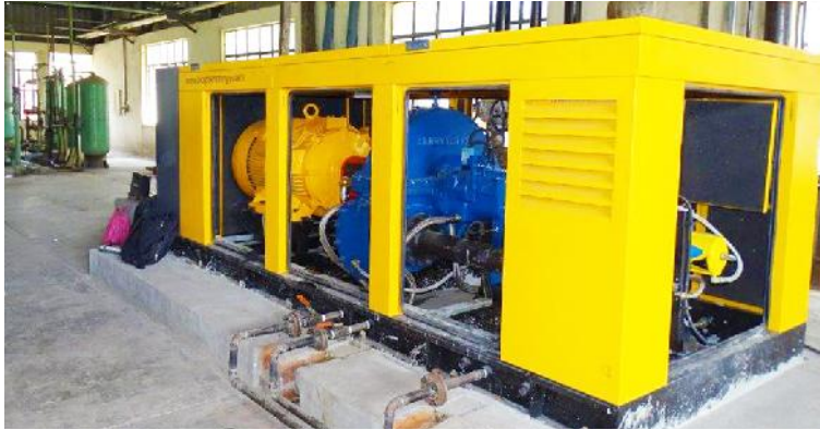
At Malanpur, we commissioned a 150 kW micro-turbine. This will help us convert pressure loss in steam lines into power, generate 100 kWh of power per annum.
