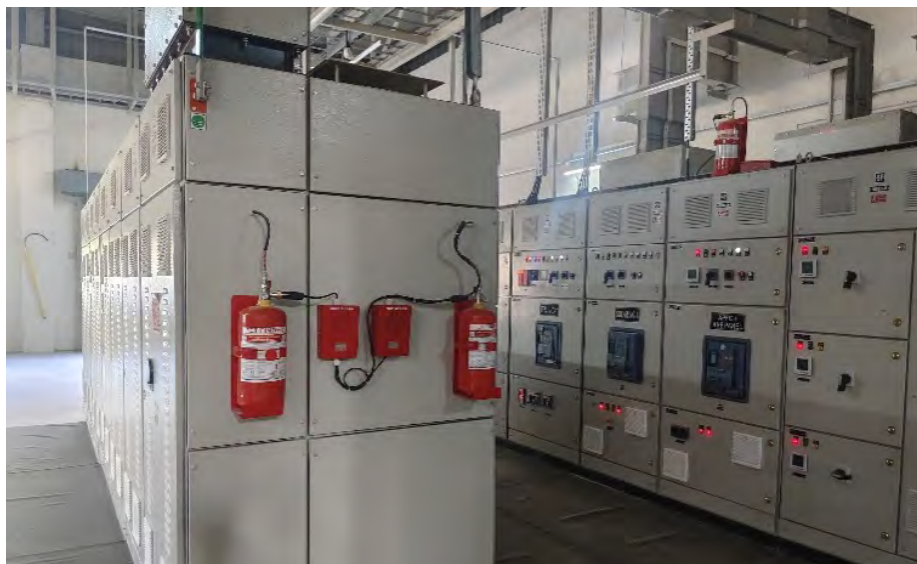
Panel for Fire protection
