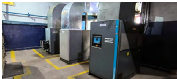
Advance Auto Energy Efficient Compressor
