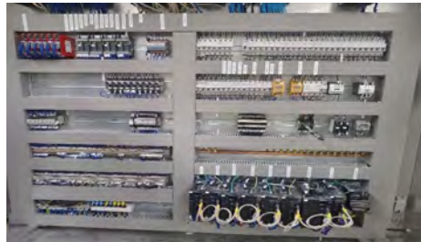
Panel with RCCB & overcurrent protection
